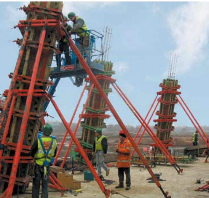
Raking column forms – Mercedes Benz Heritage and Technology Centre, Brooklands, Weybridge, Surrey (courtesy Peri)
