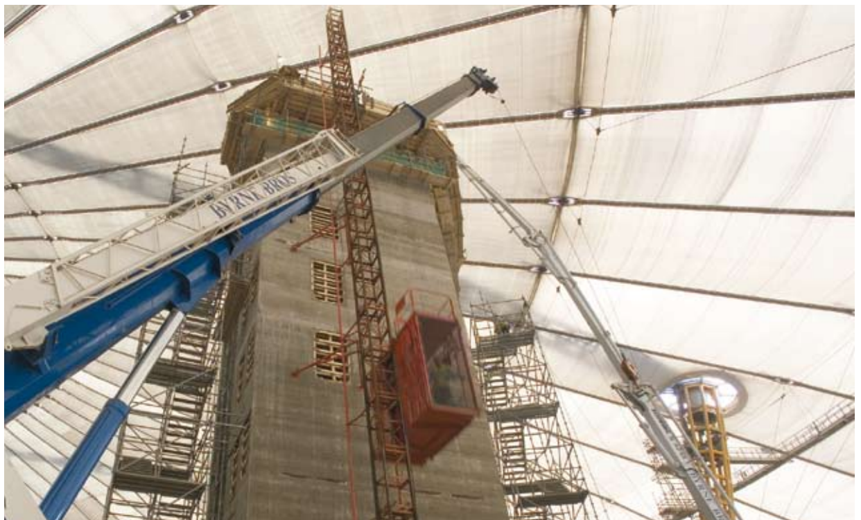
Slip form core for the O2 Arena, Millennium Dome, London (courtesy Byrne Bros)
