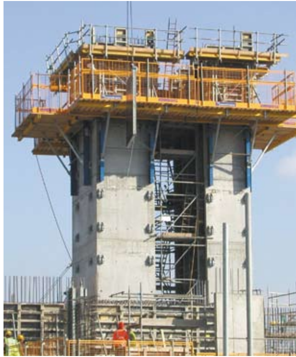
Guided climbing formwork for the core of Riverside Quarter residential development Wandsworth, London (courtesy Doka)
