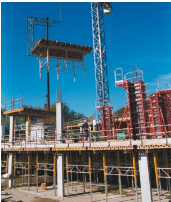
Moving table forms using a C-hook, and proprietary column formwork incorporating access platforms (see pages 18–19) (courtesy Peri)
