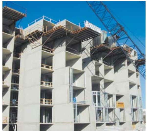
Tunnel form at Allen Street Apartments, Dallas, Texas, USA (courtesy Outinord/G Hendoux)
