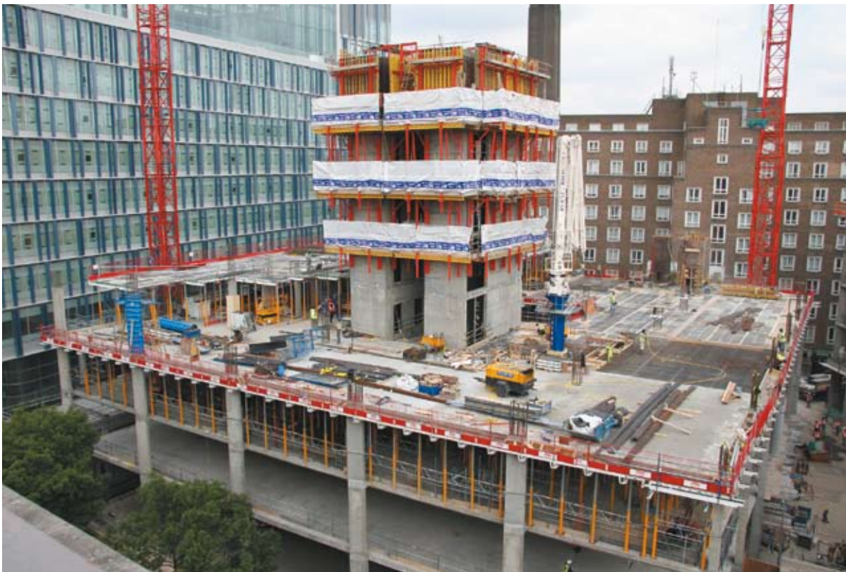
Mixed office/retail/leisure development at Bankside, Southwark, London using rail-guided climbing formwork for the core, with lightweight panel system for flat slabs (courtesy Peri)
