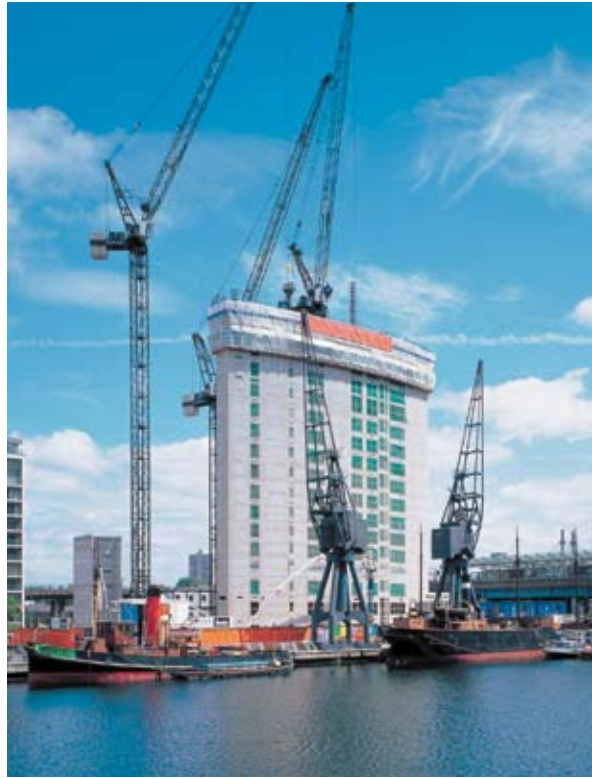
West India Quay, Canary Wharf, London – slip form core (courtesy PC Harrington)
