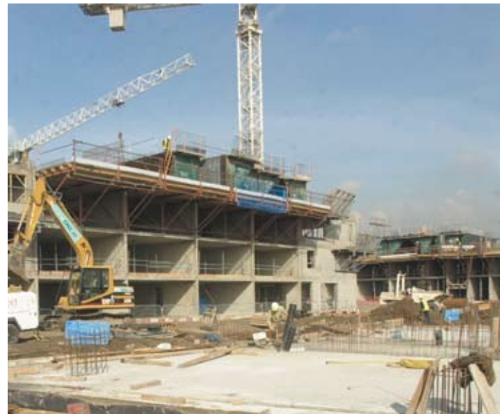
Queen Mary student village, University of London – tunnel form structure (courtesy Outinord/G Hendoux)
