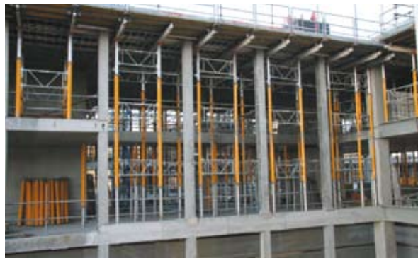
School of Informatics, University of Edinburgh using lightweight panel system (courtesy Peri)
