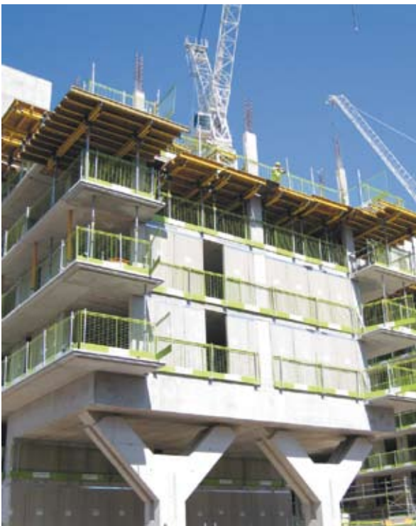
Completed jump form core and table form for a residential development, Manchester (courtesy Doka)
