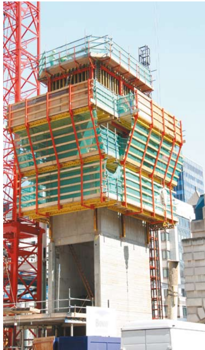
Climbing formwork system for the core of Royex House, Aldermanbury Square, London (courtesy Peri)
